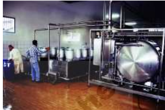
Fig-7 Chilling center
