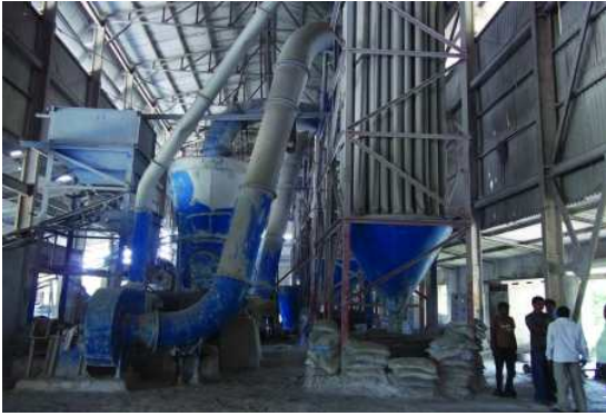
Fig 6.12: Crushing and packing plant
